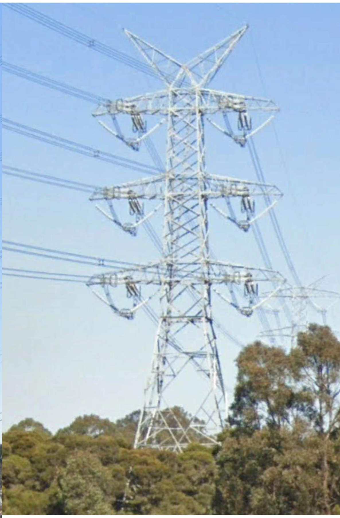
500kV Small Angle Tension Tower
