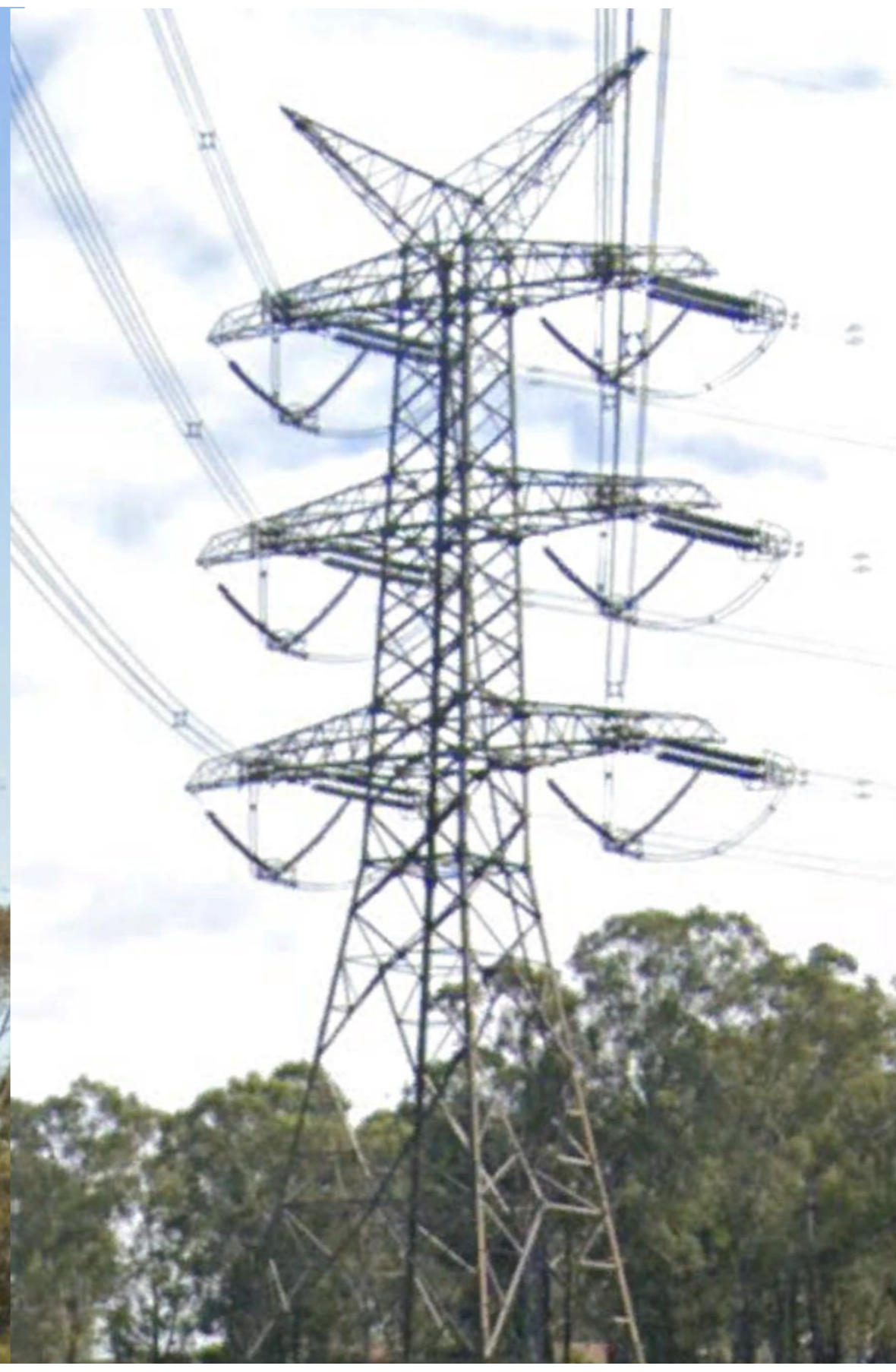
500kV Heavy Angle Tension Tower
