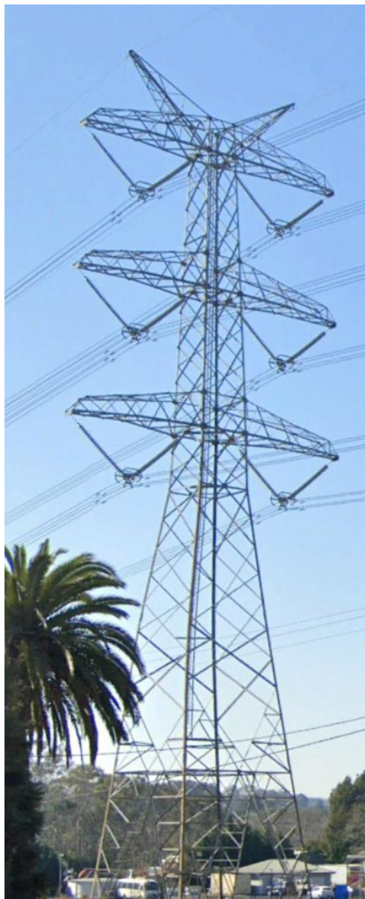
500kV Suspension Tower
