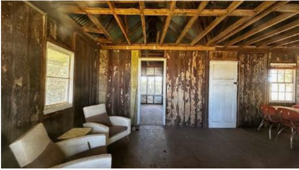
Plate A.51 Cottage looking north into extension, note newspapers on timber walls
