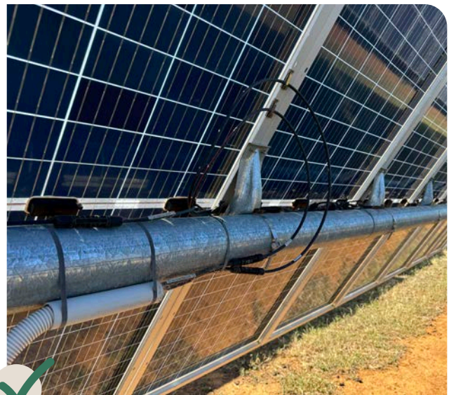
Wires inaccessible to sheep
