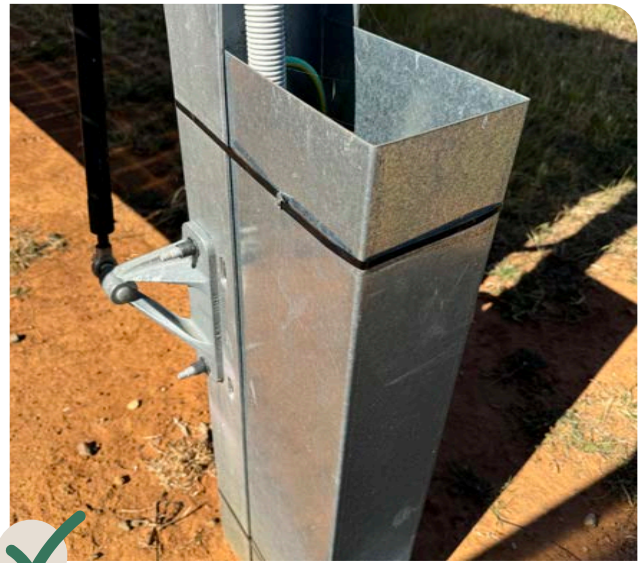
Protective guard to prevent sheep damage
