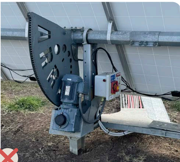
Exposed equipment accessible to sheep
